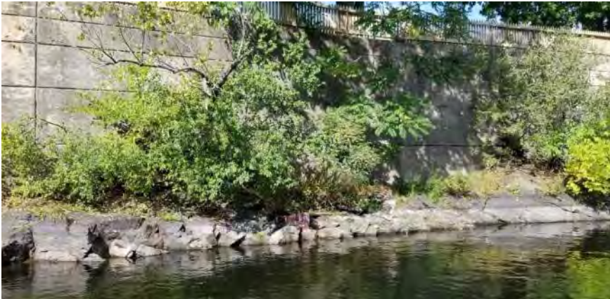
Polygon No.: 70 Photo No.: 70 Date: 9/26/2019 Direction Photo Taken: Northwesterly Description: The canal wall is primarily concrete with trees, such as locust and elm, growing at the toe of the wall.
