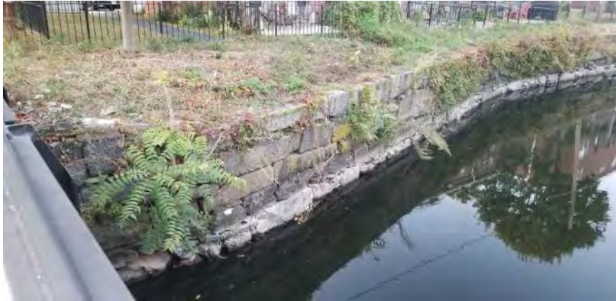
Polygon No.: 39 Photo No.: 39 Date: 9/25/2019 Direction Photo Taken: Northerly Description: A few small tree of heaven trees are growing out of the canal wall, near the top of the wall.
