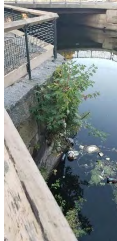
Vegetation Point No.: VP-11 Photo No.: VP-14 Date: 9/26/2019 Direction Photo Taken: Southwesterly Description: A small clump of silver maples are growing out of the canal wall.
