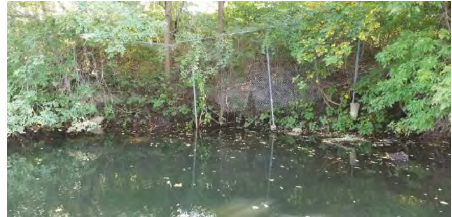
Photo Location No.: P-4 Photo No.: P-15 Date: 9/26/2019 Direction Photo Taken: Easterly Description: Dense vegetation is growing on earthen banks along the canal.
