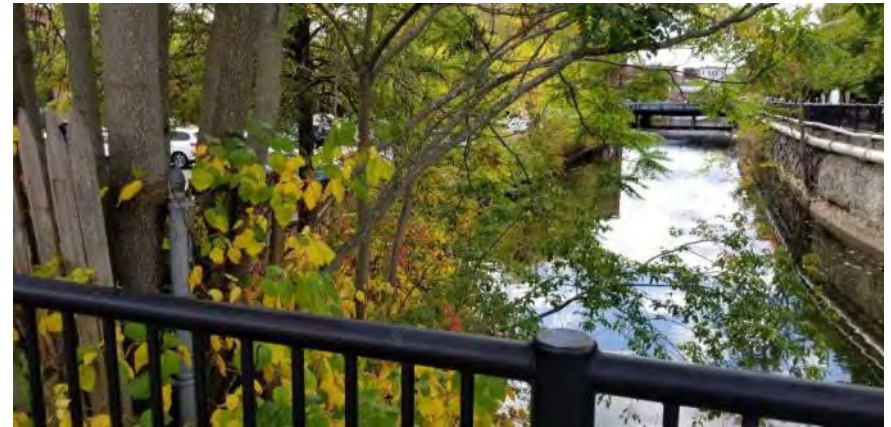
Polygon No.: 89 Photo No.: CV_Poly9 Date: 9/25/2019 Direction Photo Taken: Southeasterly Description: The vegetation growing out of the canal wall includes an approximately 10-trunked tree of heaven tree at approximately 6 inches diameter at breast height and poison ivy.
