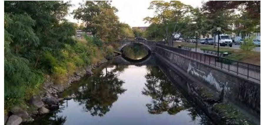
Photo Location No.: P-3 Date: 9/25/2019 Direction Photo Taken: Southwesterly Description: Vegetation is growing on the riprap shoreline located on the eastern side of the canal (left side of the photograph). The western side of the canal wall (right side of the photograph) is concrete with little to no vegetation present.
