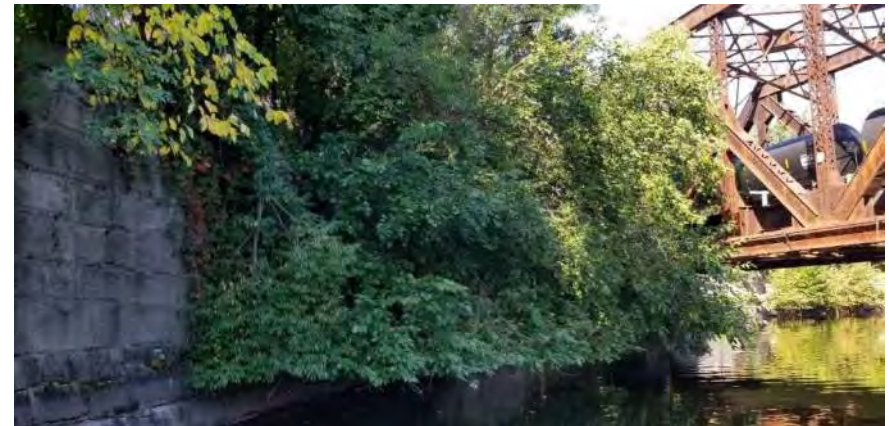
Polygon No.: 67 Photo No.: 67 Date: 9/26/2019 Direction Photo Taken: Northwesterly Description: Large locust and birch trees are growing on top of the canal wall.
