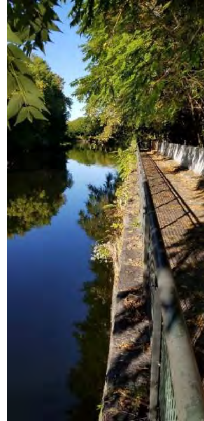
Polygon No.: 78 Photo No.: 78 Date: 9/27/2019 Direction of Photo Taken: Westerly Description: Vegetation growing out of the canal walls include tree of heaven and mulberry and herbaceous species such as purple loosestrife and mullein.
