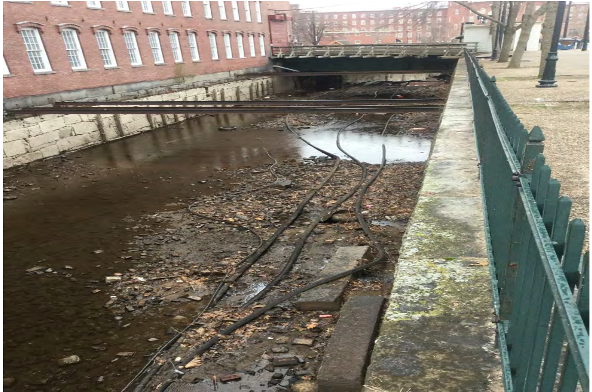
Photo 5-8. Substrate trash on bottom of Eastern Canal across from Boott Cotton Mills Museum and Tsongas Industrial History Center.
