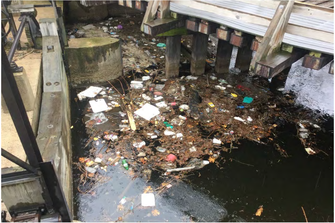
Photo 5-5. Waterborne trash on the Merrimack Canal at Market Street.
